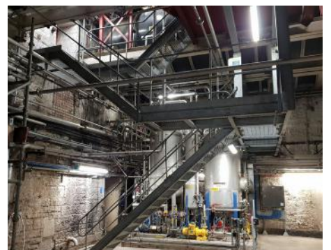
LED Luminaires in Situ - Multi Level
