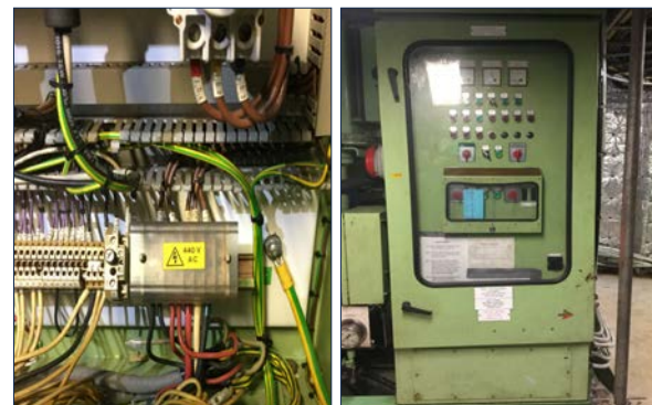
Original Diesel Engine Fire Pump Control Panel
