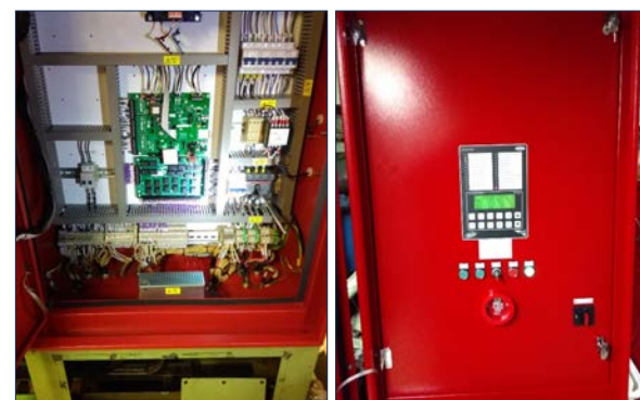
Replacement Diesel Engine Fire Pump Control Panel
