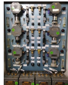
Overhauled aspirated panel
