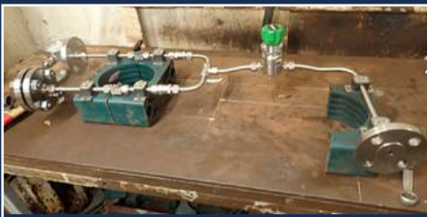
Preparation and Pre Fabrication Testing of the Flare Tip Package Detection Components
