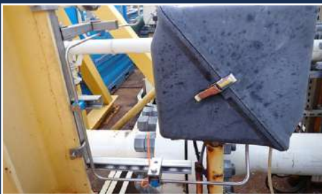
Gas Decoupling Control System Header to PT Enclosure
